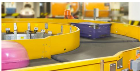
Airport baggage handling
